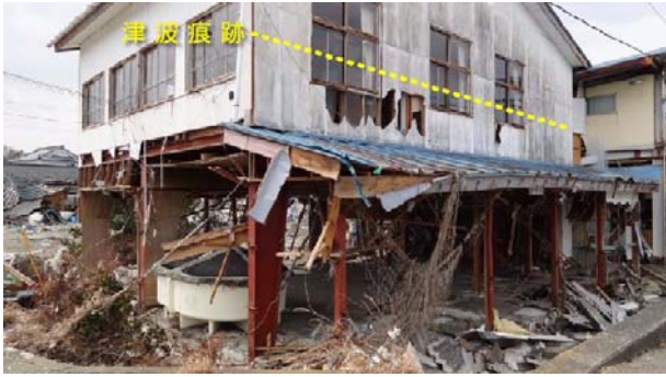
図8 花渚漁港の建物の被害. Fig. 8 Damage of a harbor building at Hanabuchi fishing harbor.
