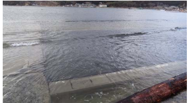
図16 牡鹿半島桃浦地区の港の被害. Fig. 16 Damage of a harbor at Momonoura hamlet of Oshika Peninsula.
