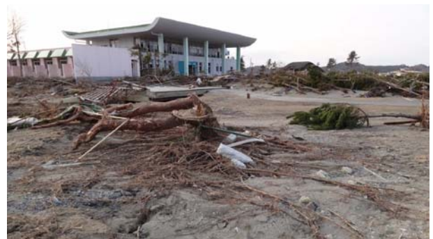
図11 東松島市野蒜の松島自然の家の被害. Fig. 11 Damage of Matsushima gymnasium at Nobiru, Higashimatsushima City.
